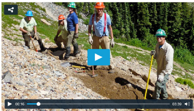
WTA volunteers working on a trail reroute at Easy Pass, in the north Cascades (Photo by Barbara Eller)
