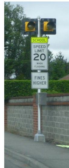
Figure 3. Clark County School Zone Speed Limit Flasher System
