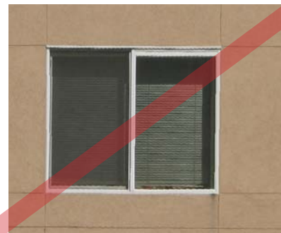
Figure 6-39. An example of unacceptable window design.
