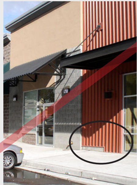
Figure 6-45. Masonry or concrete would be required within 2 feet of ground for this metal sided storefront.
