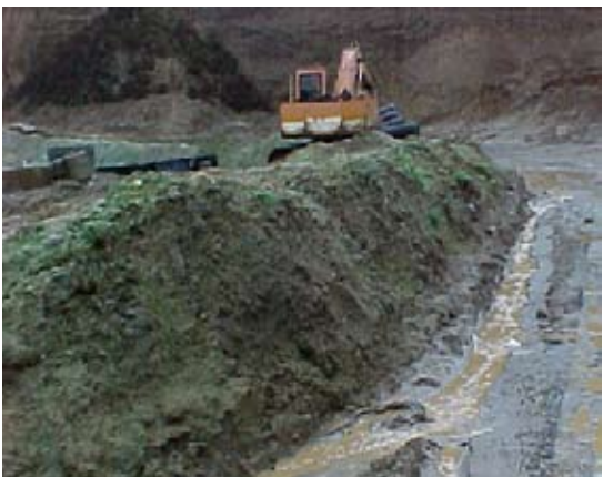
Turbid runoff into Mud Lake stopped through the joint efforts of Clark County, Washington State Department of Ecology, and the business operator.
