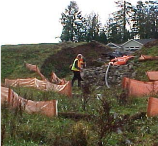
Inspectors check stormwater facilities and work with the owners to correct problems.
