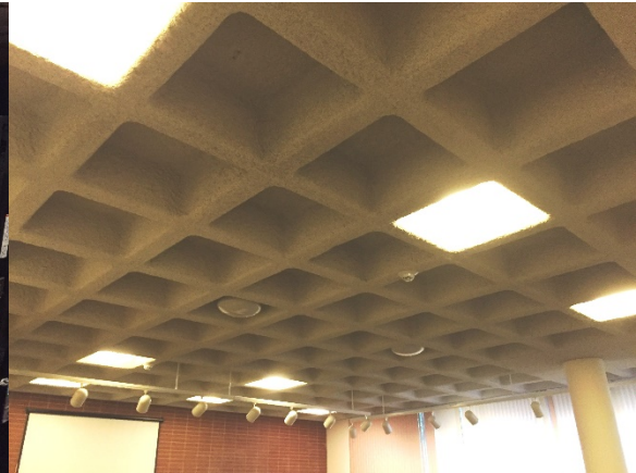
Example of waffle slab from meeting area. This is similar to the waffle slab referred to in the loading area.
