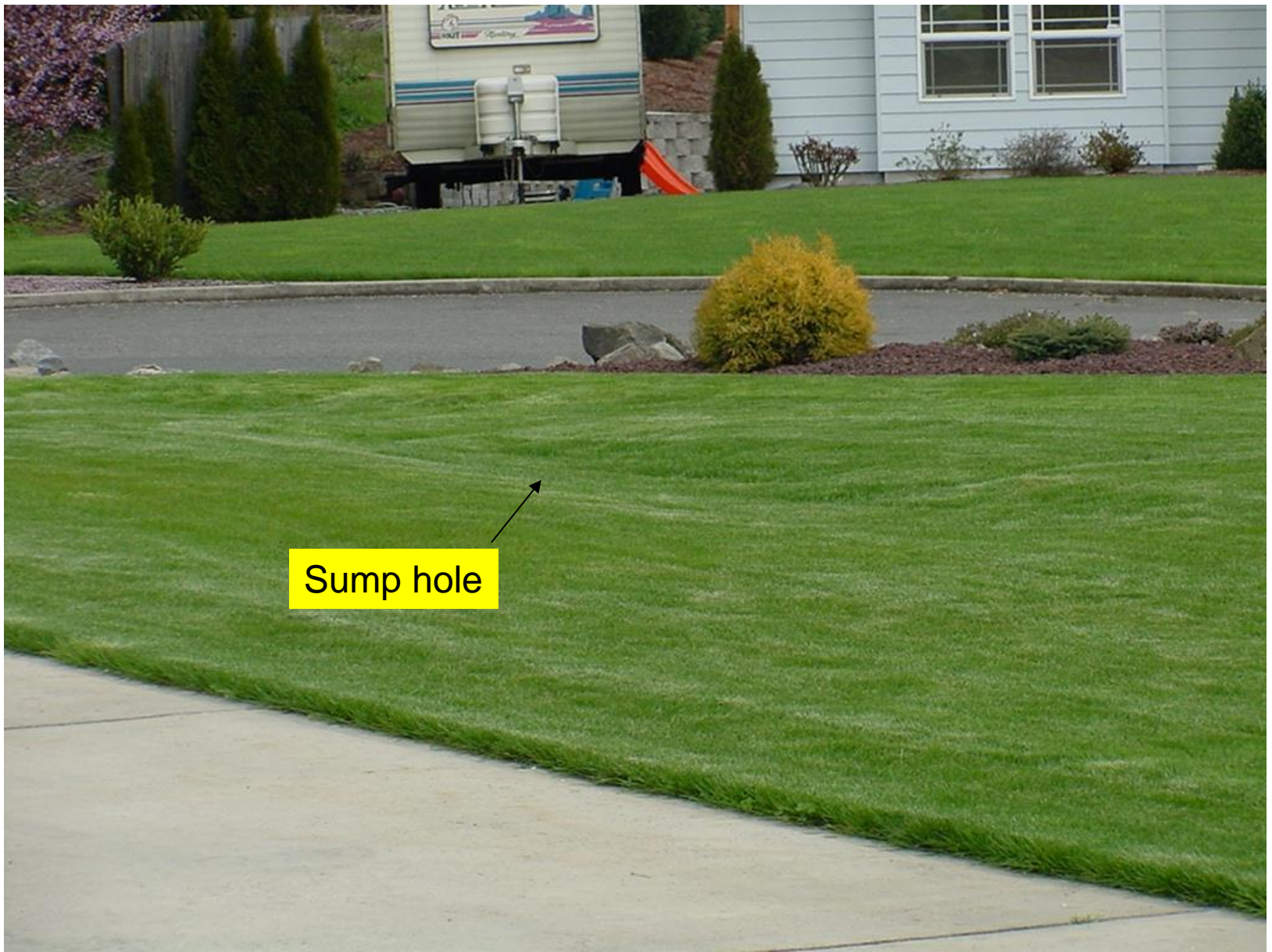
This area sunk about a year after they filled the sink-hole in the street. It took about 10 trucks of dirt to bring it back to level.
