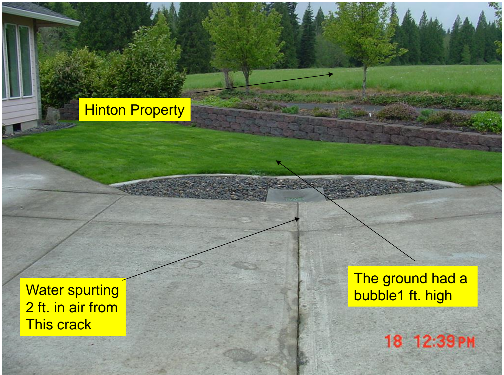
This is after the second fix. The first fix was a 3" pipe. The next good rain caused the ground to bubble up a foot and water to fountain up 2' along this crack.
