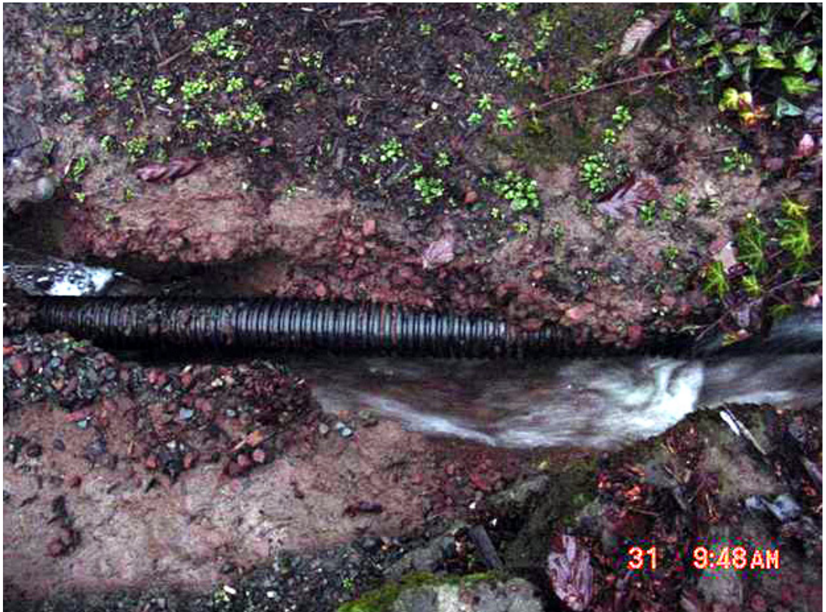
In places the erosion is 18" deep from water the drain pipe could not handle.
