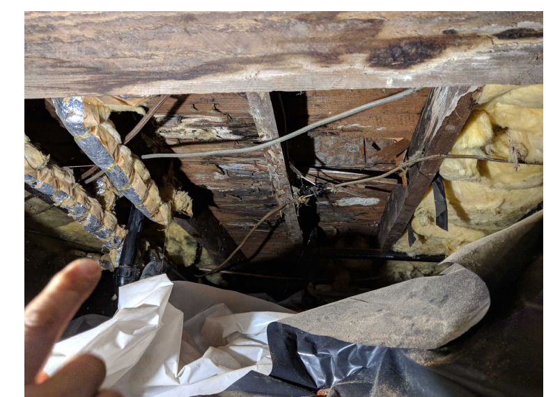
A PHOTO - ROTTED FLOOR JOISTS
