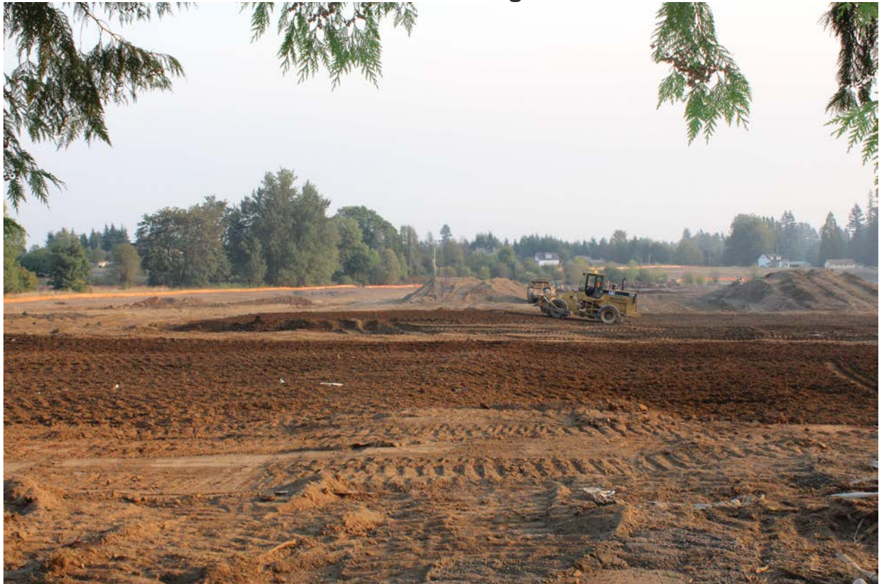
The construction of the Cedars Village Subdivision at the Cedars Golf Course at Salmon Creek is underway. Site preparation began this spring for 117 lots on the 39 acre site which encompasses the driving range and holes one and two. The photo was taken September 14 th from behind the club house looking south. Holes one and two are being reconfigured. The new driving range is in the planning stage.
